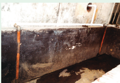
Heat Treatment water tank
