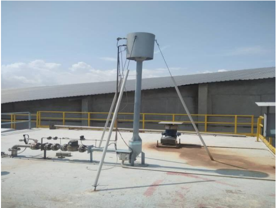
WWTP Biogas Production- Flaring
