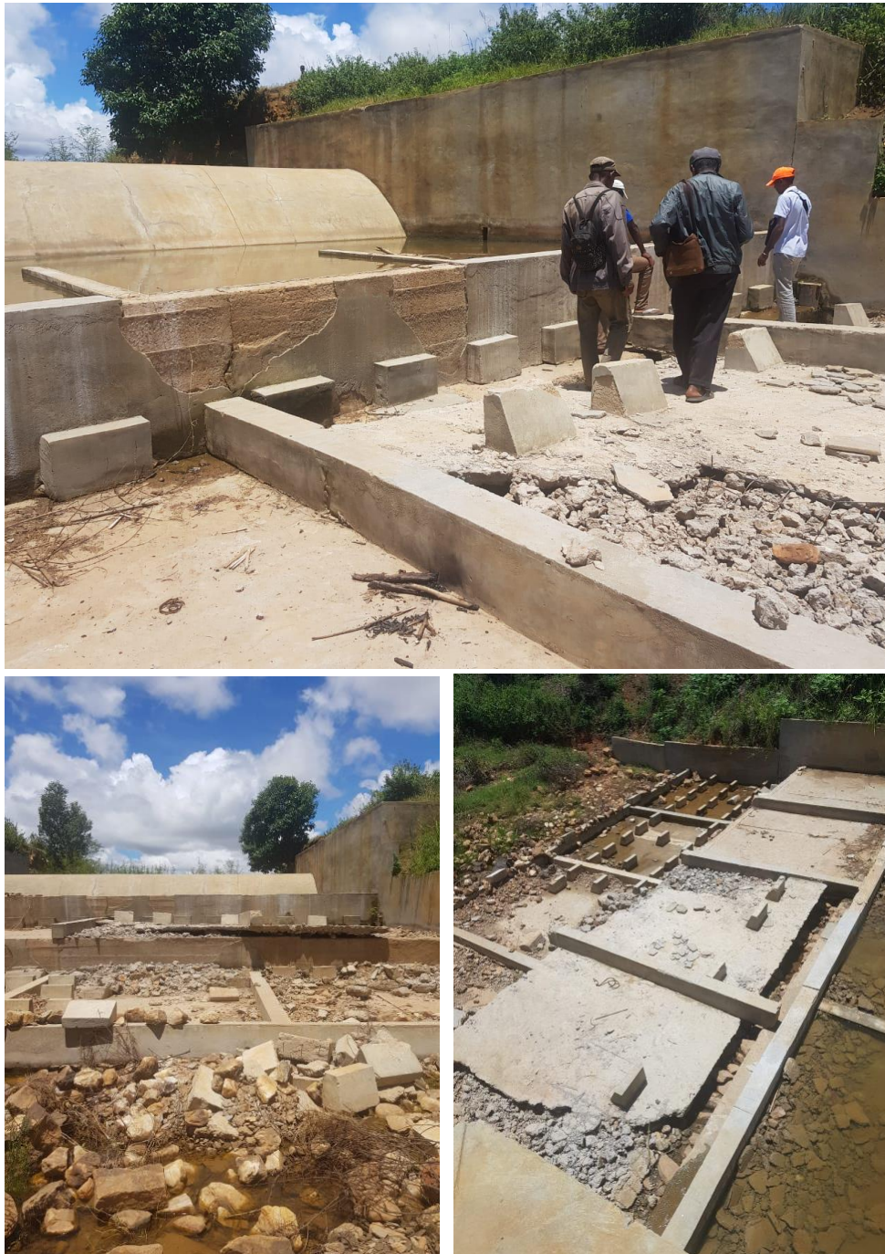
Figure 10. Damaged spillway in Bemaïtso.
