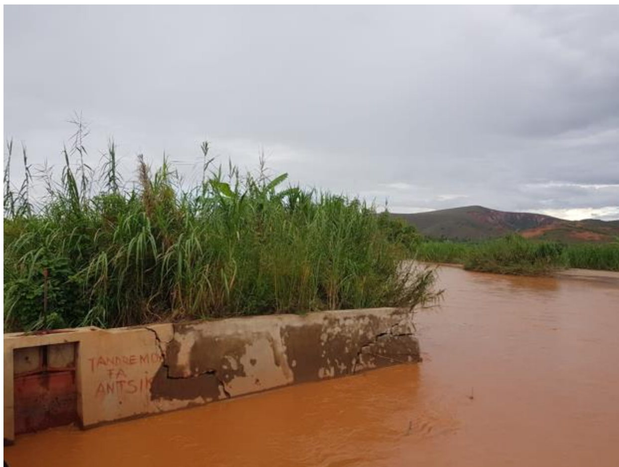
Figure 6. Damaged main water intake in Manakambahiny.
