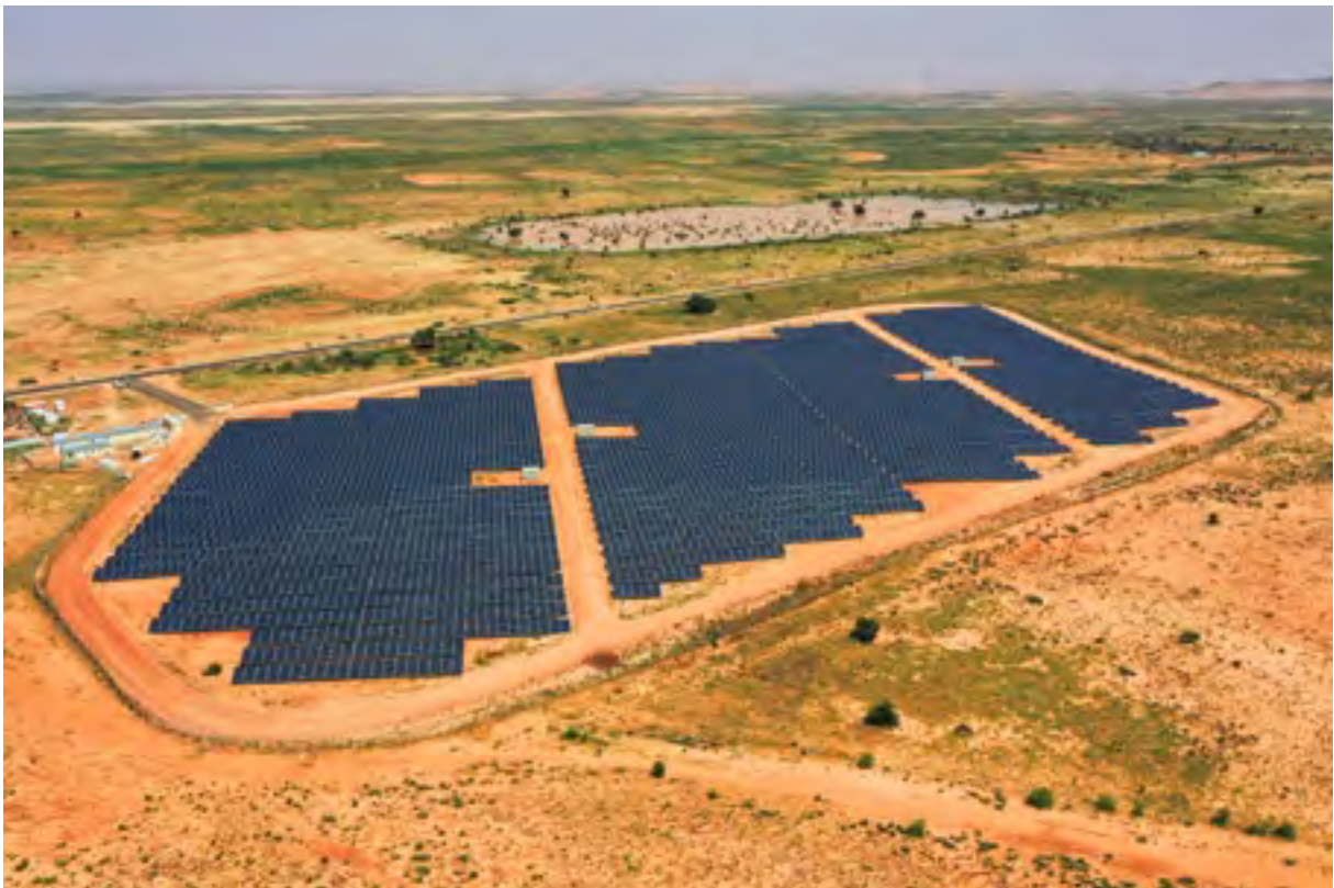
Sudan’s future energy policies should boost investment in clean forms of energy such as the solar energy station in North Darfur. Photo credit © UNEP
