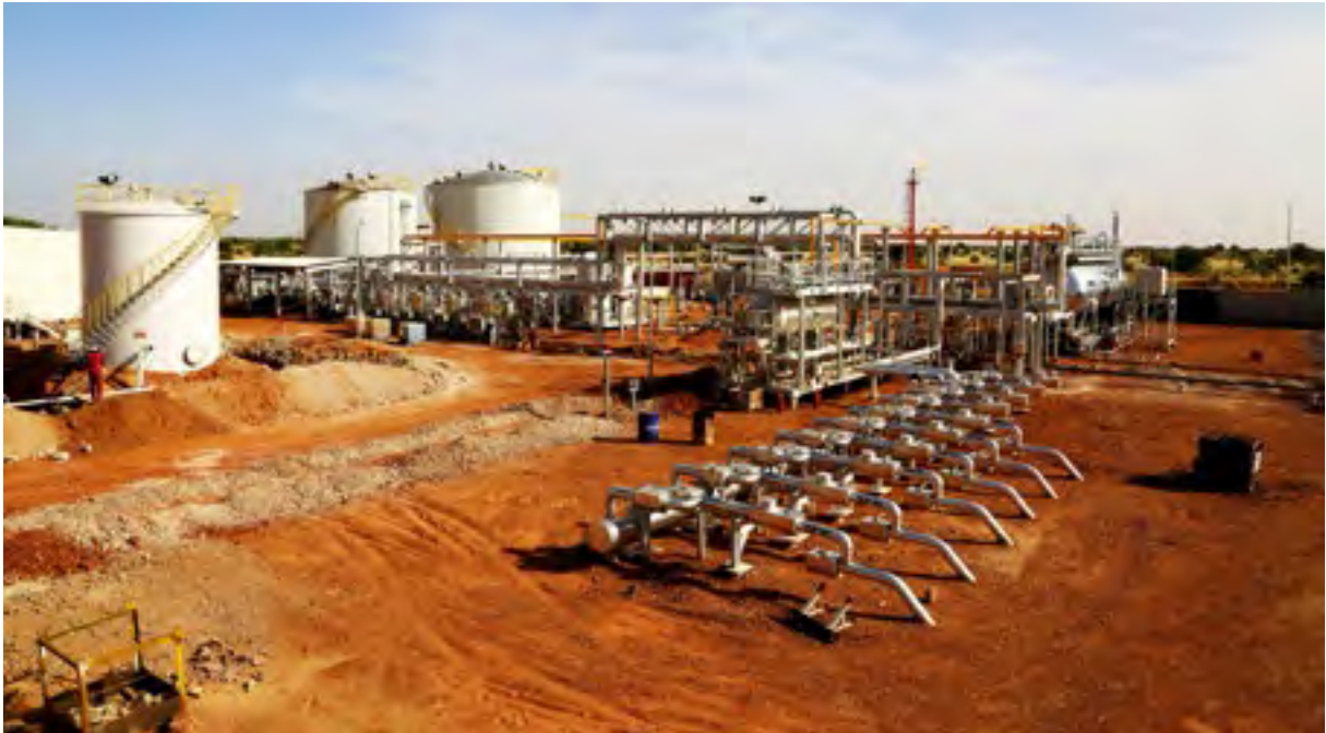
Despite the loss of 75 per cent of oil reserves in 2011 due to the secession of South Sudan, oil is still an important resource in Sudan. Photo credit © UNEP
