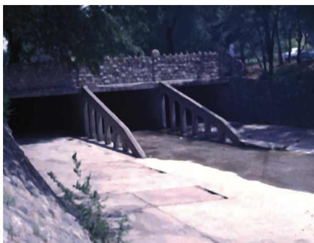
Figure 14. Concrete debris fins extending upstream from a bridge pier
