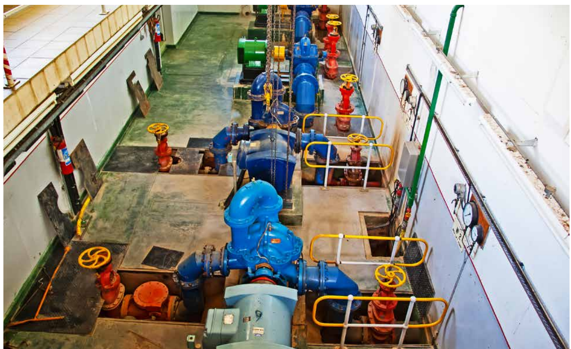
The low electricity generation capacity in many African towns and cities negatively affects wastewater treatment
