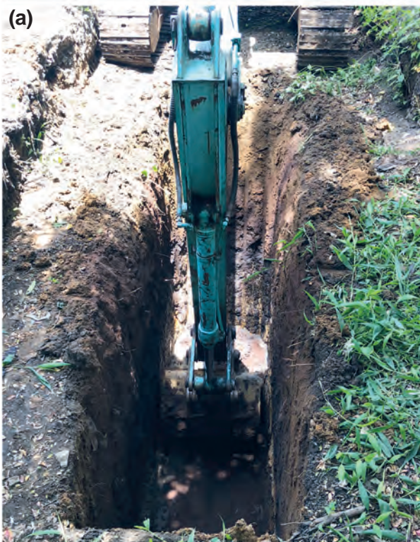
a) Trench excavation across the groundwater flow paths to install PRB materials (1 m wide, 5 m deep and 60 m long) at Sundarapola dumpsite, Kurunegala, Sri Lanka
