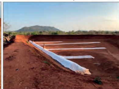
Leachate pipe with geotextile
