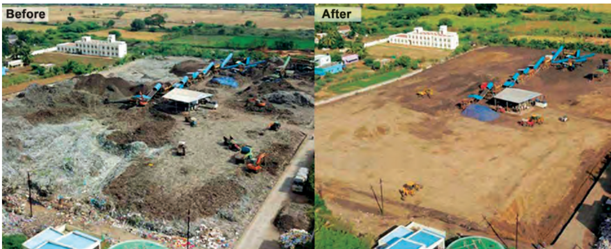
Figure 9.2 Stabilization of legacy waste in the dumpsite; (right) reclaimed land after completion of biomining process (CSE, 2020)
