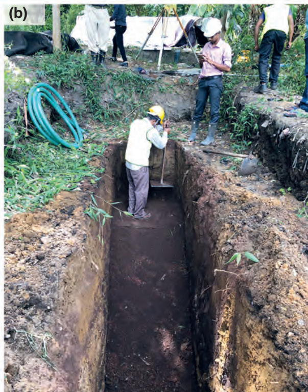
b) Trench filling by PRB materials (Biochar+ clay brick particles + dense clay) and compaction to finish the installation
