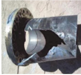
624 Figure 6. Metallurgical failure caused by mercury in a gas processing facility 625 (IPIECA).
