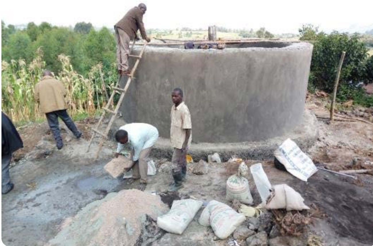
A community rainwater harvesting water tank under construction in Nzogera village ©Water for Virungas (W4V)
