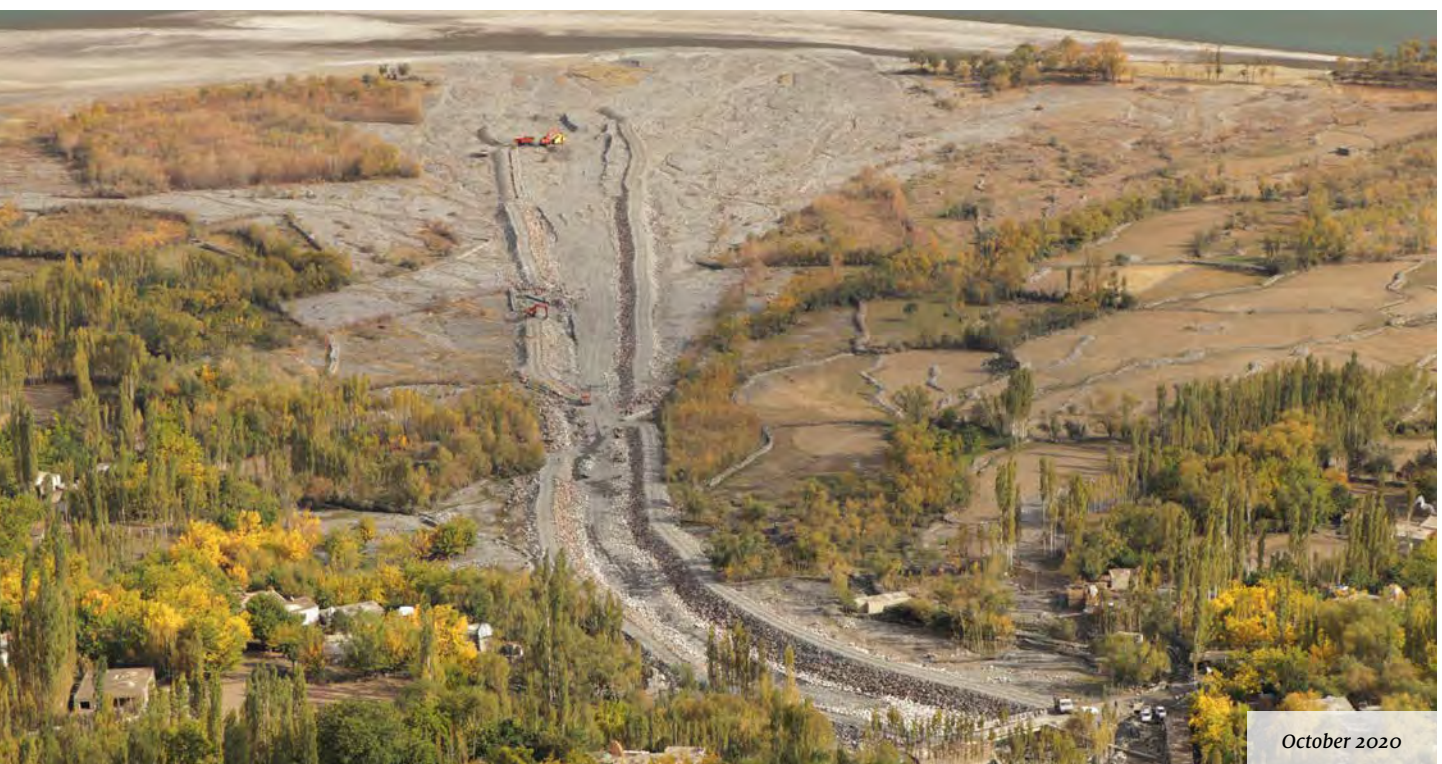
Deh-Shahr alluvial fan before and during construction of the new flood protection dyke
