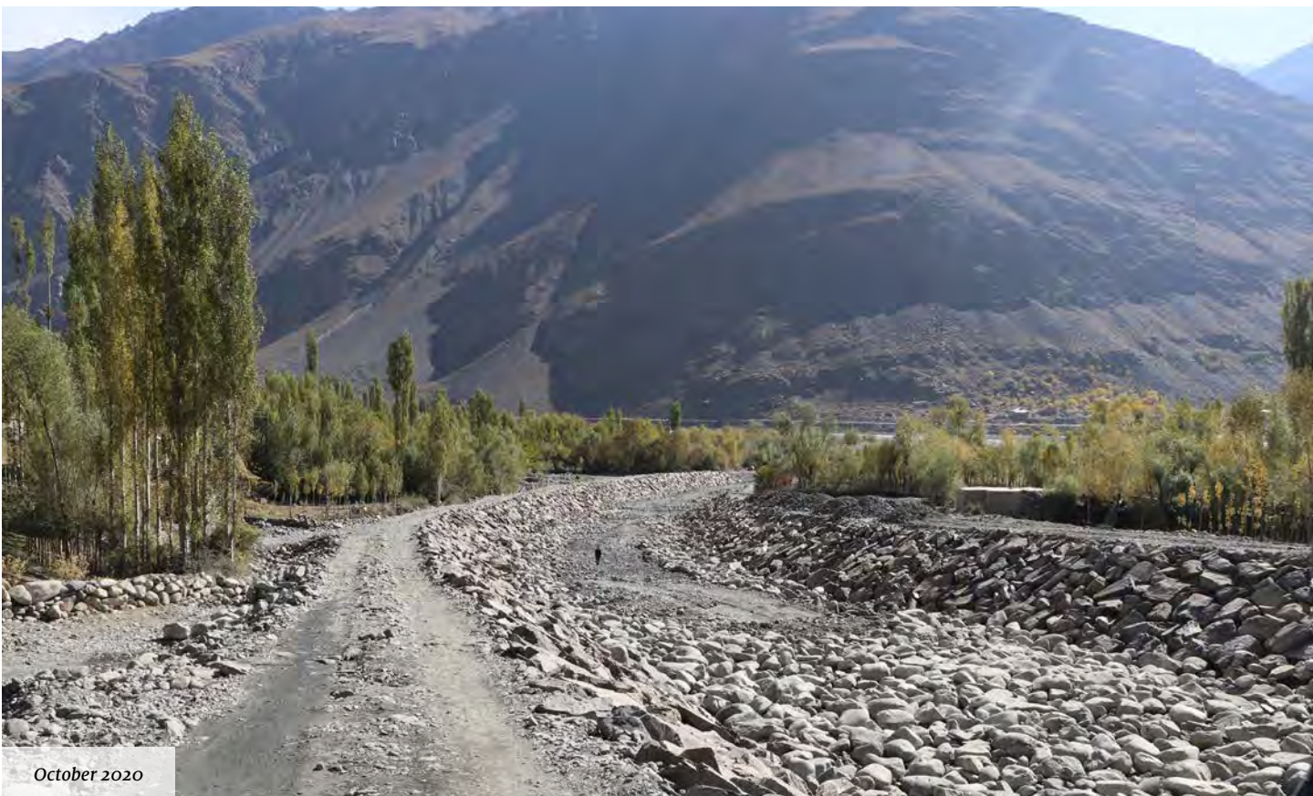
An on-the-ground view of the old and new flood protection dyke of Deh-Shahr alluvial fan
