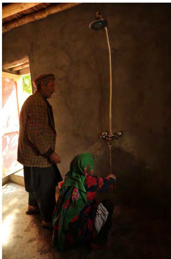
A beneficiary equipped his bathroom with a shower system to capitalise on use of solar water heaters
