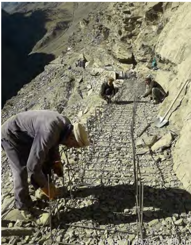
Community members working to connect the Oshtuk mountain irrigation canal after cutting through the rocks
