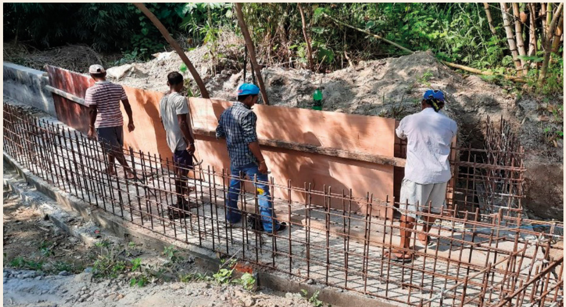
Community members contribute to water infrastructure maintenance in the Karnali River Basin, Nepal
