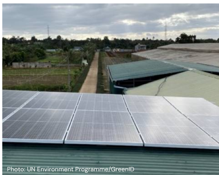
In Photo: Water pumps running on power from solar PV system benefit women farmers
