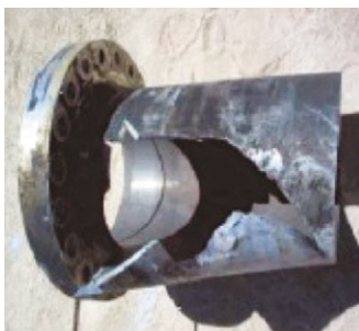
FIGURE 5: METALLURGICAL FAILURE CAUSED BY MERCURY IN A GAS PROCESSING FACILITY (IPIECA) 80
