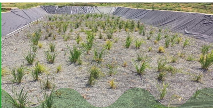
The Shimo La Tewa waste treatment plant under construction, July 2022. Photo credit: Kenya Marine and Fisheries Research Institute.
