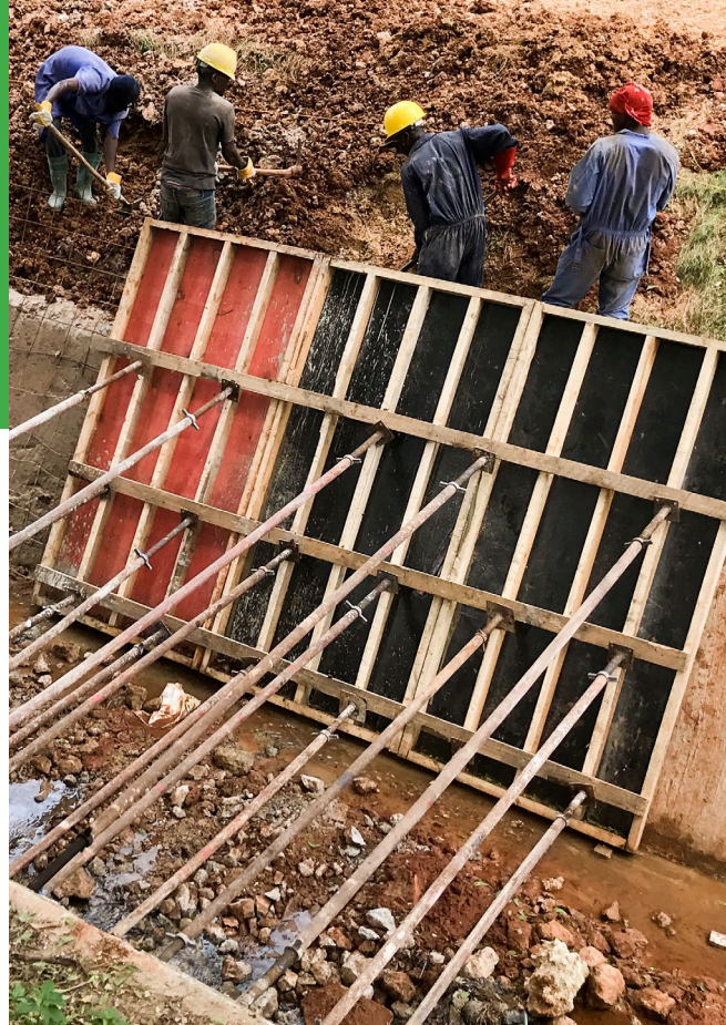
People can now get fresh water from wells that had turned salty due to sea water intrusion, thanks to a mangrove resforestation project supported by UNEP in the Kisakasaka community in Zanzibar. Photo credit: UNEP
