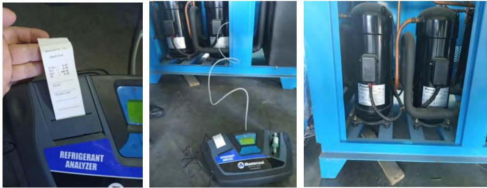
Seizure of one chiller at the customs post in Sergeli/Tashkent on 6 November 2019
