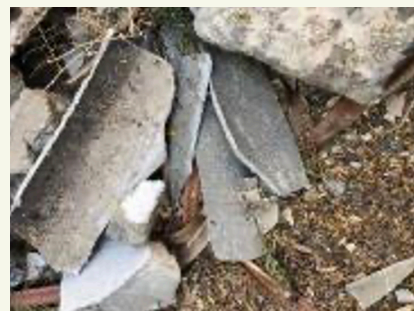
Figure 1: asbestos containing materials within general debris
