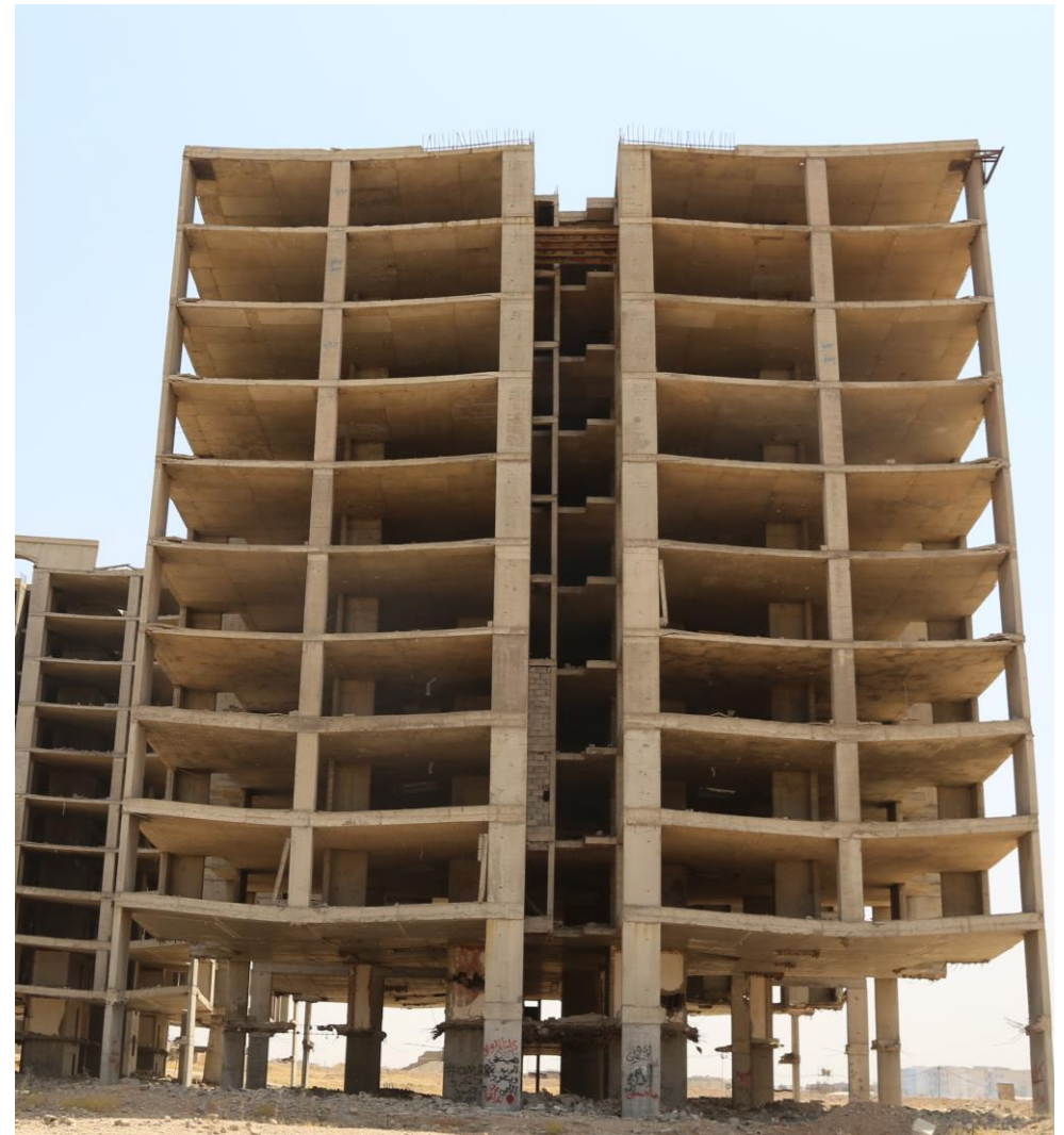
Photo 5: The demolition of these 10-storey buildings – visibly denting inwards after ISIL blew-up their foundation beams - will generate a considerable amount of rubble.
