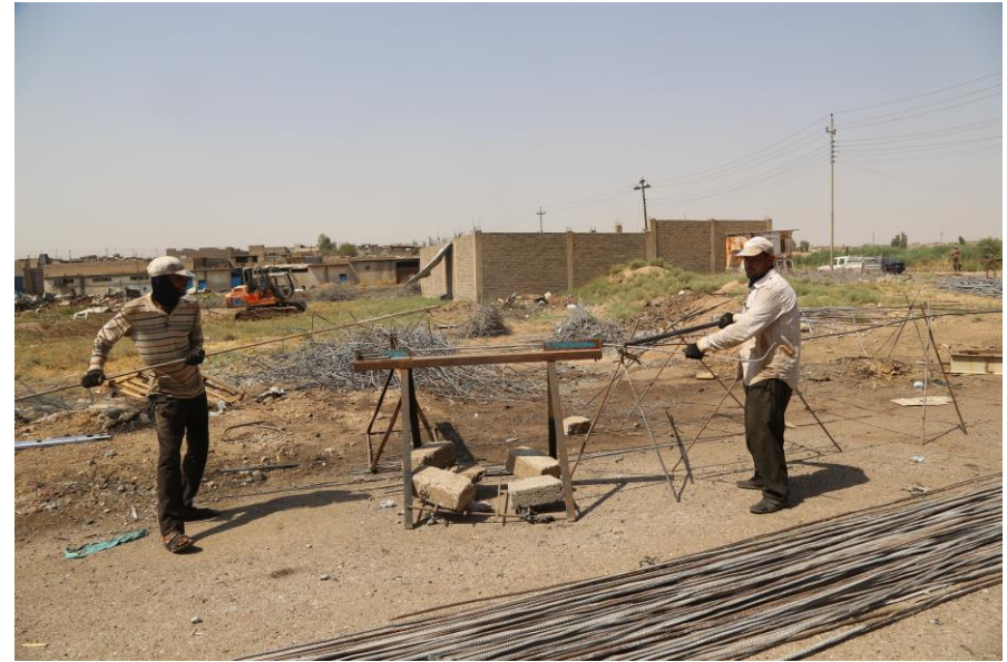
Photo 11: Recovery of reinforced steel bars from rubble is a source of work in Mosul
