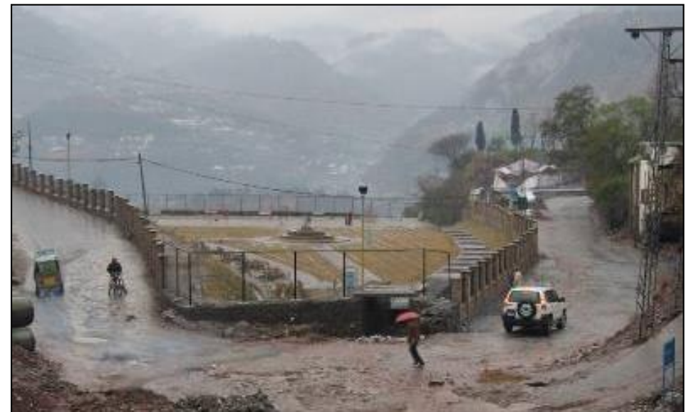
Photo 9: Debris recovered as part of clean-up operations in Muzaffarabad (Pakistan) was used as engineering fill material
