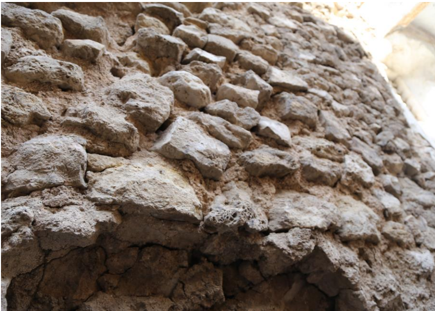
Photo 3: Extensive use of gypsum and lime in the construction of Old City buildings may limit the recycling value of the debris
