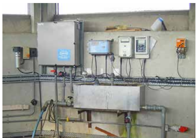
Figure 7.2 Continuous monitoring of water quality at a drinking water treatment plant intake tower. Water from the intake gate is diverted through a tank in which the sensors are placed. The outputs from the sensors are relayed to a control room, where the information is used to decide on depth of abstraction and level of treatment required © Deborah Chapman
