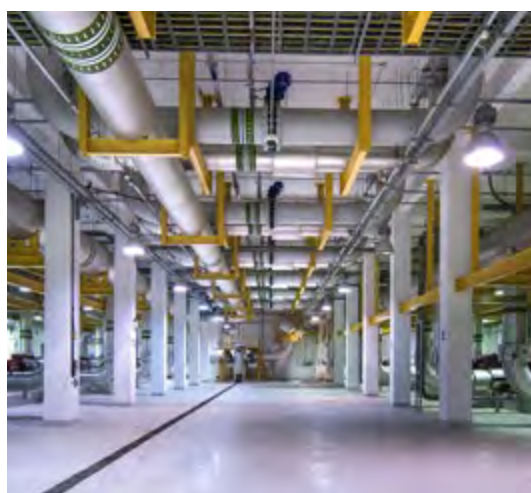
District cooling plant Photo: Plamen Galabov, shutterstock
