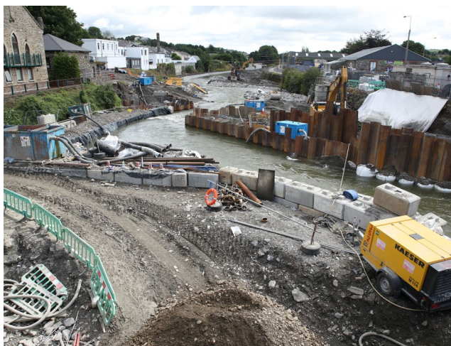
Figure 1.1 Flood protection works on the Bandon River, Cork, Ireland creating major hydromorphological alterations to the river – destroying benthic habitats and increasing suspended solids. © Patrick Cross
