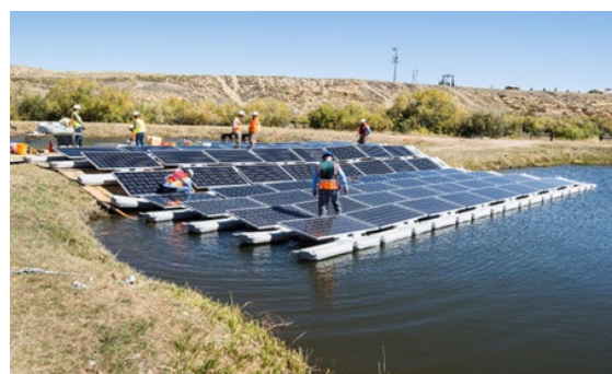
FPV Installation in Walden, Colorado (National Renewable Energy Lab)
