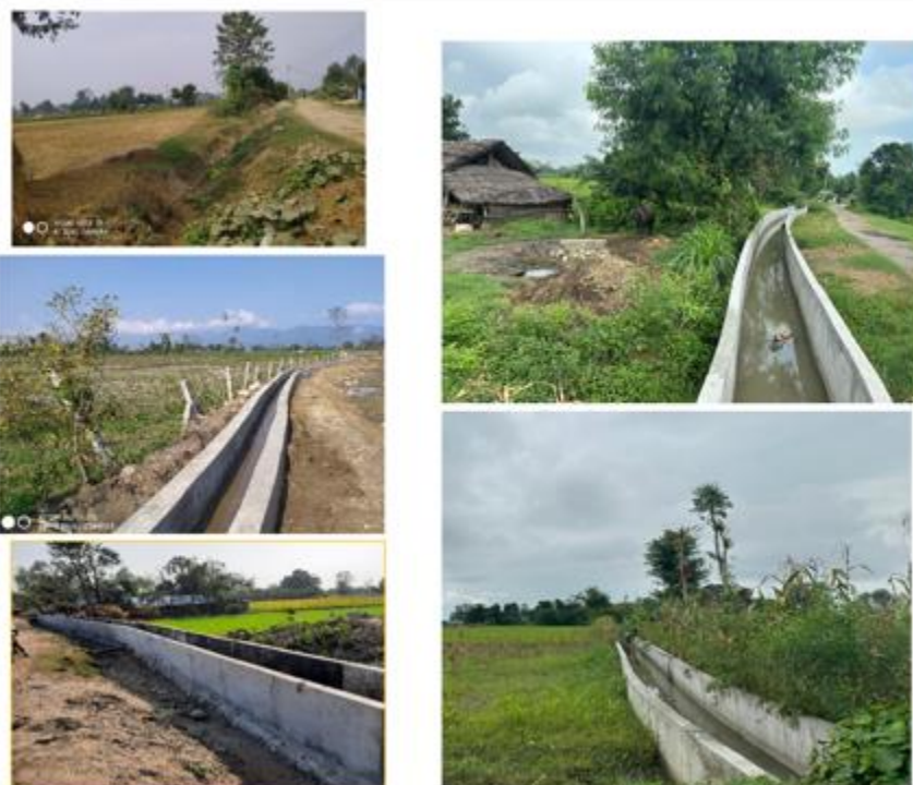
Figure 14 RCC wall construction works in Nepal (before and at the time of TE)
