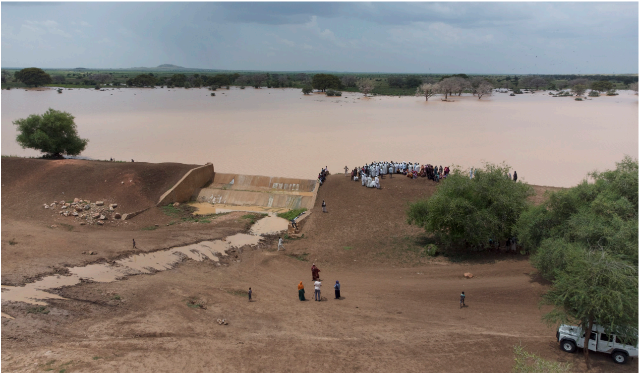
Wada'a dam underwent rehabilitation despite Sudan's conflict in mid-April 2023. It was fully operational during the rainy season and brought positive impacts on drinking water, farming, and the environment. Photo credit ©UNEP
