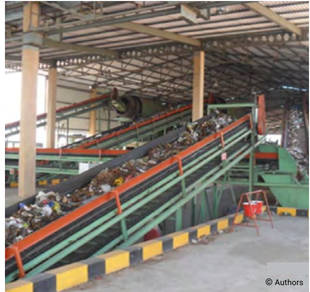
Figure 13: A conveyor system at a facility
