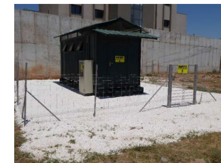
Mercury Storage Container
