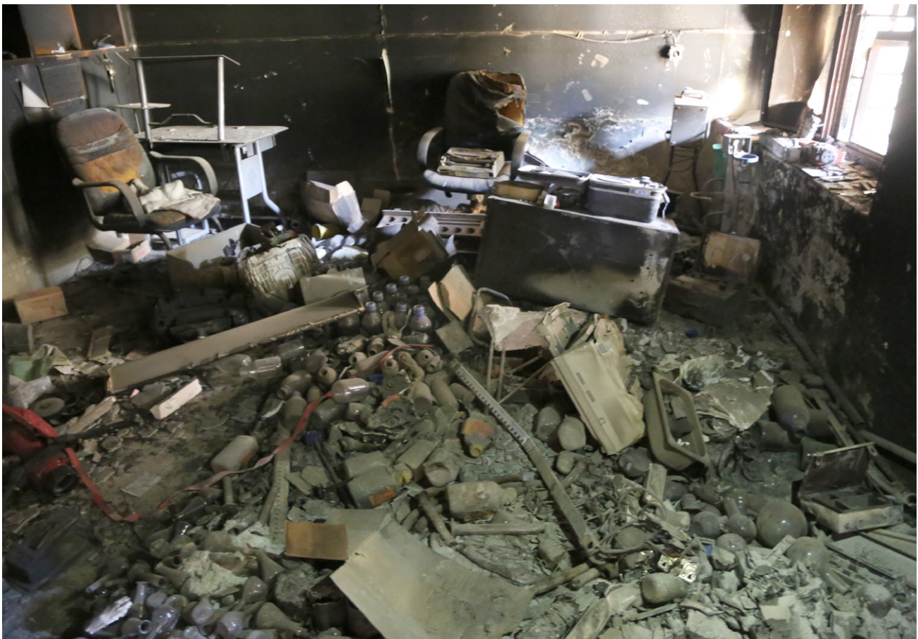
PHOTO 8: The offices of the Niniveh Environment Directorate in Mosul were destroyed during the ISIL conflict
