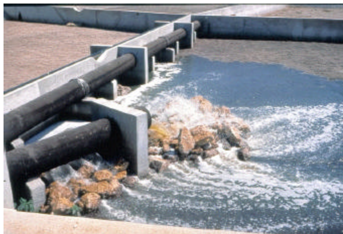
Figure 3.12. Flush feeding of an infiltration percolation basin
