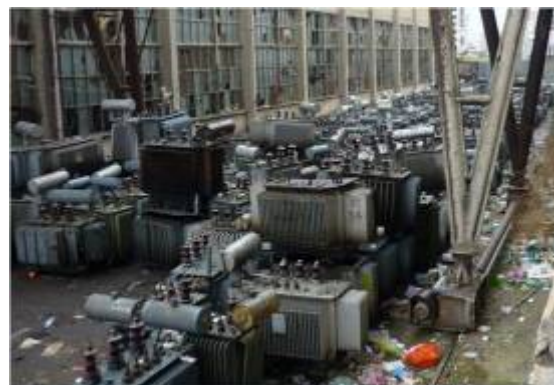
Photo 8: Transformers containing PCB contaminated oil in electrical companies inspected in 2010
