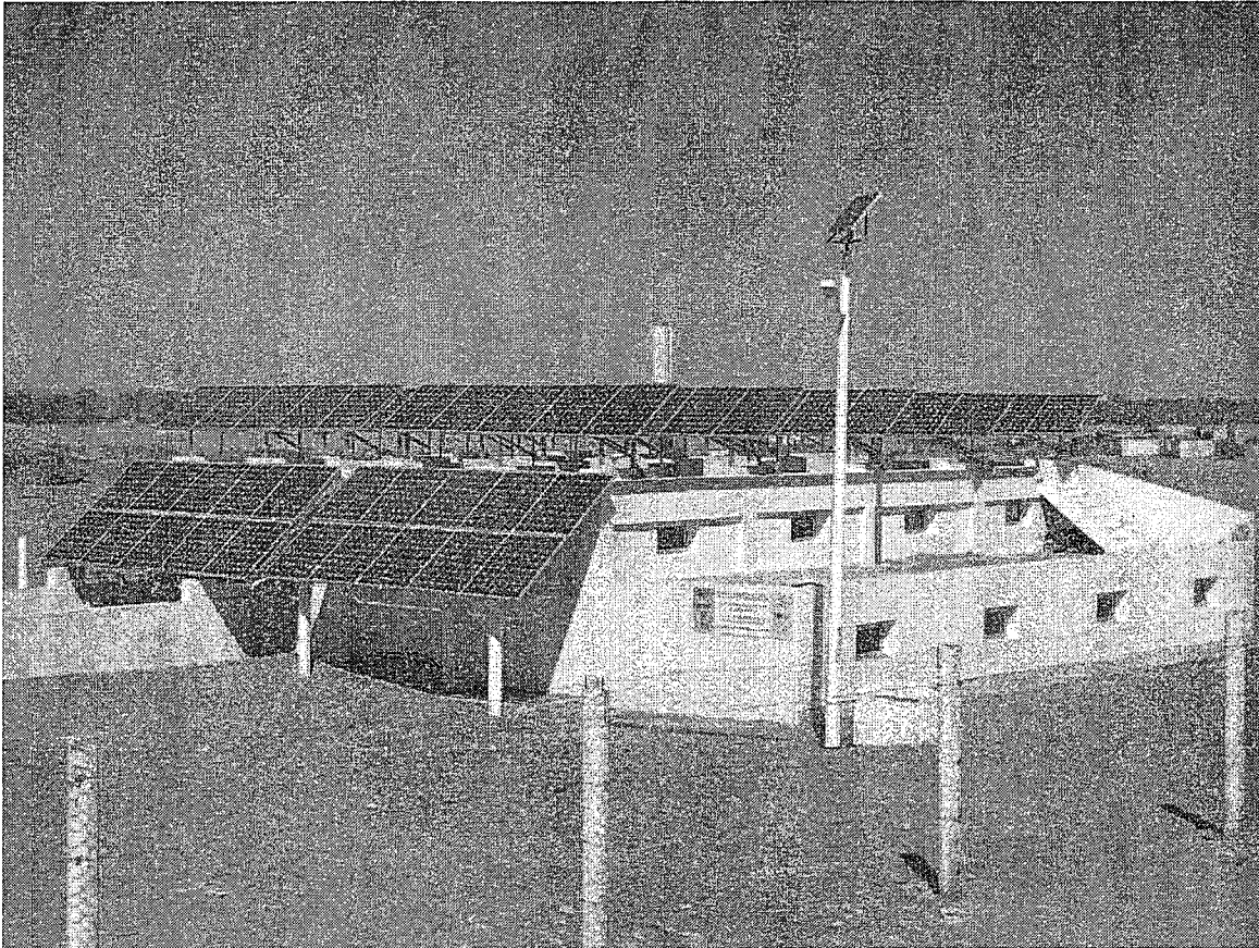
Figure 23: A 2.1 m 3 /h nominal capacity brackish water PV-RO plant in Tunisia, installed by the Canary Island Institute of Technology, Spain.
