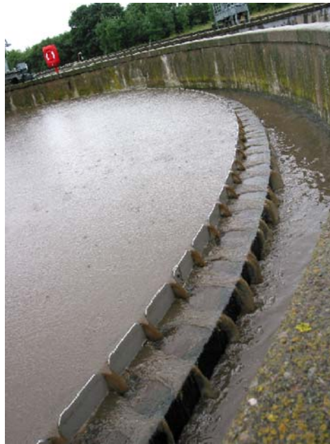
Figure 3. View of poor solid removal of a primary settler due to hydraulic overloading with storm water
