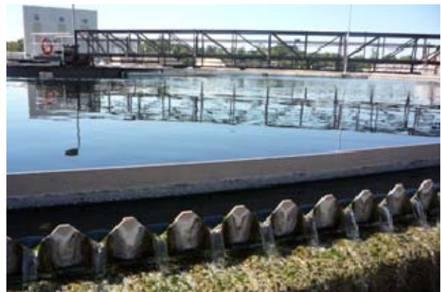
Figure 2. View of a primary sedimentation tank
