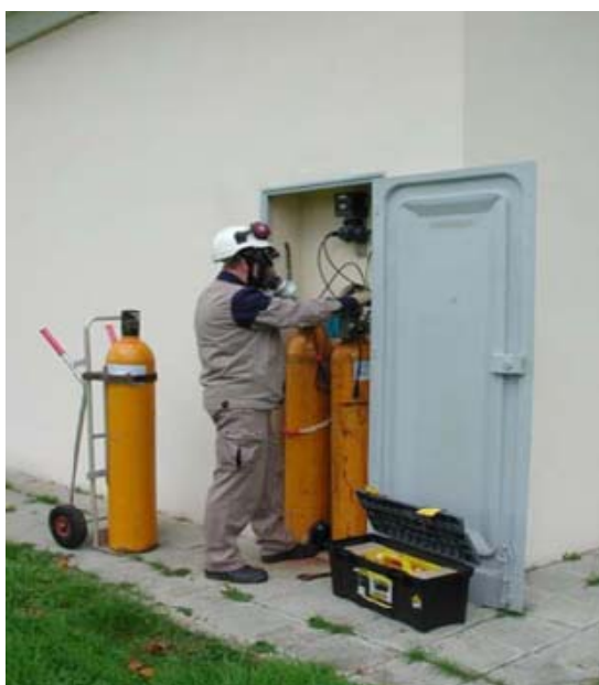
Figure 17. View of chlorine storage and handling in small facilities
