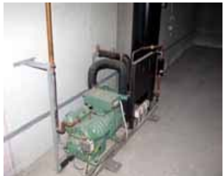
Figure 9: New Danfoss R-404 compressor at Linda Ltd.
