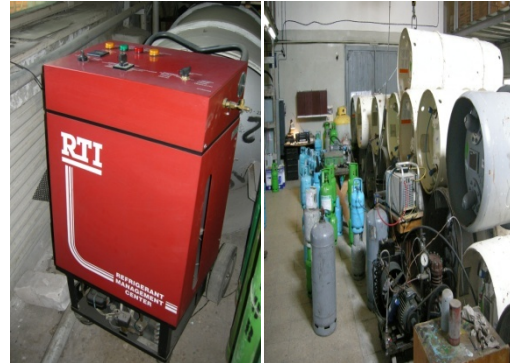
Figure 30: RTI recovery and recycle equipment (left) and stored ODS (right). Revers Refrigeration, Latvia.
