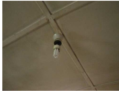
Insulated ceiling and CFL lamp installed in one of the demonstration houses.
