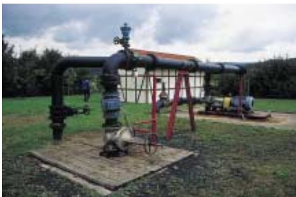
Deep well injection of brines - Kali und Salz GmbH, Germany
