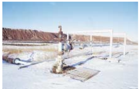
Deep well injection of brines - Potash Corporation of Saskatchewan (PCS), Canada
