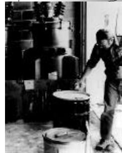
Temporary PCB storage
