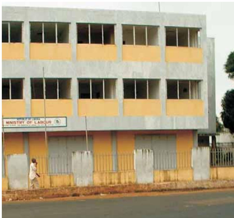
Looted Ministry of Labour building in Monrovia, December 2003
