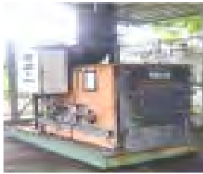
Picture 2.16.1.2 A typical retort type multi-chamber incinerator
