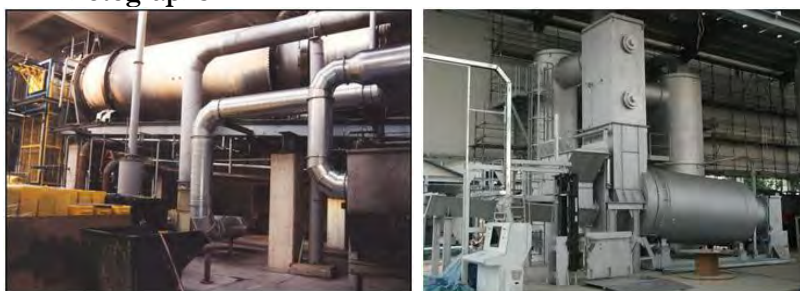
L-R: Co-current rotary kiln, counter-current rotary kiln (900 kg/hr)
