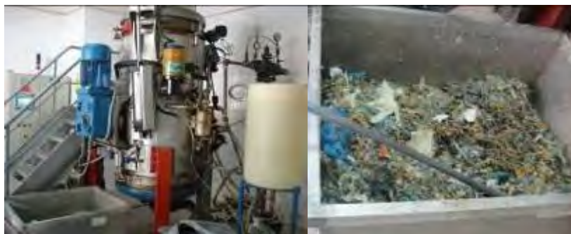
Figure 11.22. Ecodas T300 at Hotel Dieu Hospital, Lebanon
