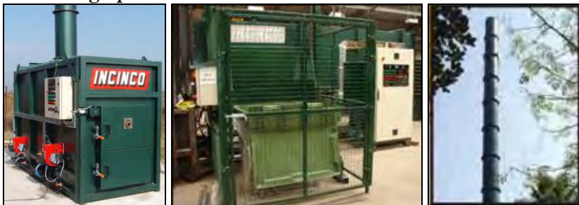
L-R: Incinco hospital incinerator, waste bin tipper and controls, hospital stack
