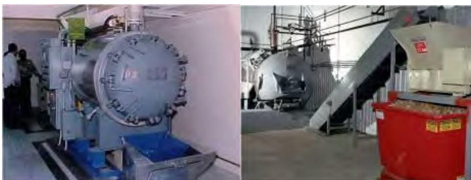
Figure 11.20. Hydroclave, conveyor and shredder at Tata Memorial Hospital, India
