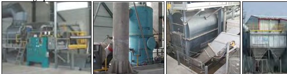
L-R: Pennram medical incinerator, wet scrubber, wet ash conveyor, baghouse filter
