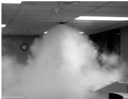
Discharge of a halocarbon system in data processing center
