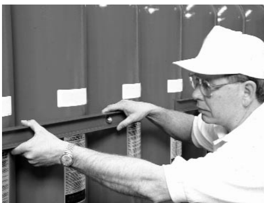
Securing an inert gas agent supply
