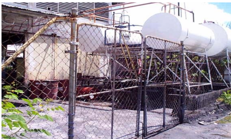
Figure: 13.3 Betio Power House in Royds, 1996 Vol 2
