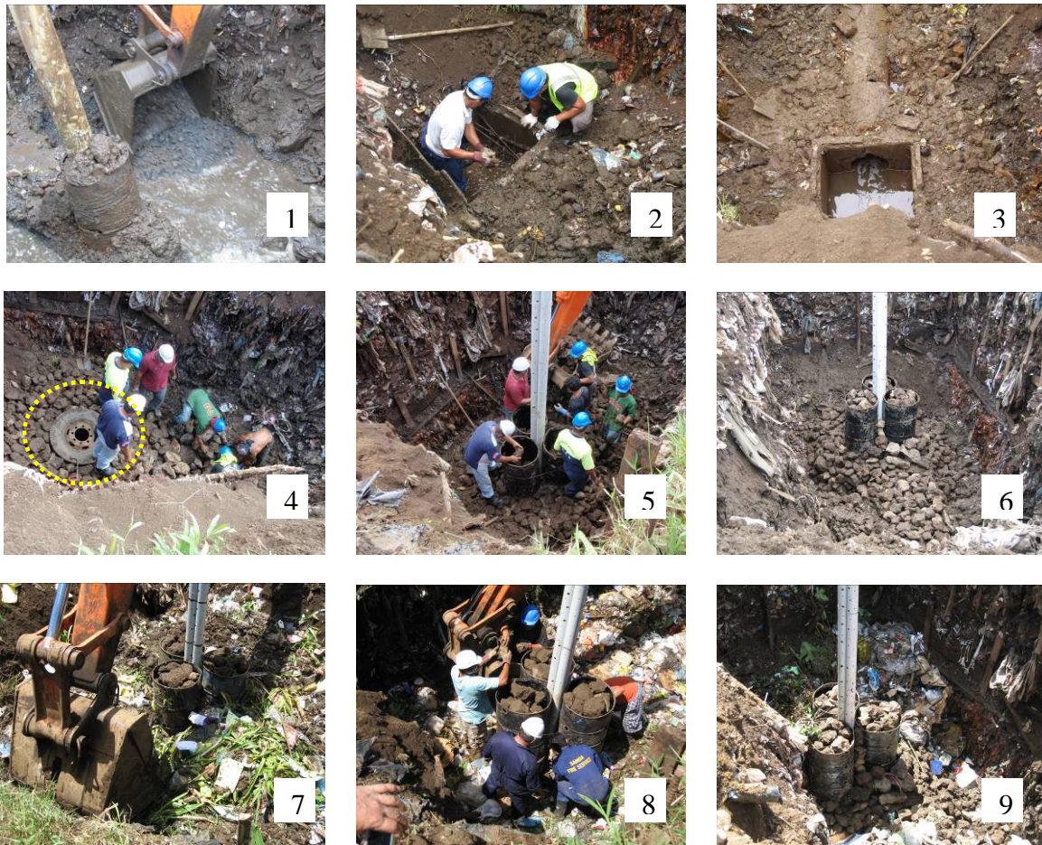
Photo- 45: Sequence of Remediation of Damaged Gas Venting Facility on the Connection Pit
