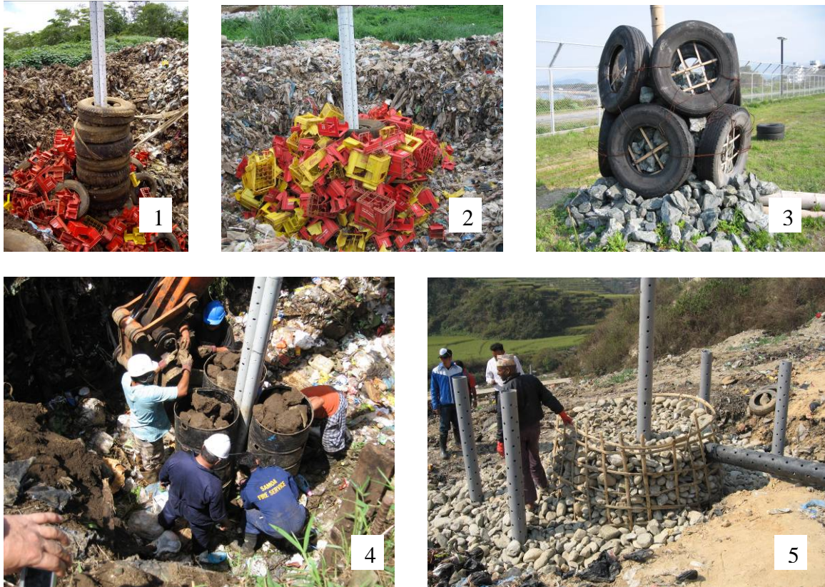
Photo- 29: Different Types of Vertical Gas Venting Facility to Enlarge the Aerobic Zone around the Pipe
