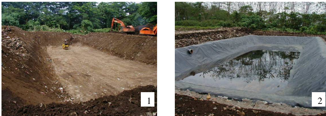
Photo- 23: Leachate Retention Pond
