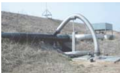
< Landfill gas supply pipes >
