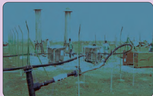
Landfill Gas Project in Malacca
