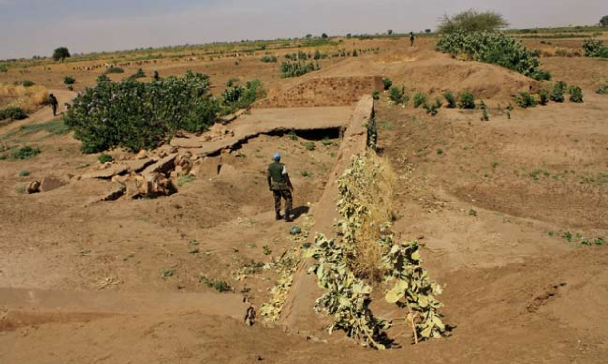
Lack of investment and conflict have left environmental infrastructure such as this weir at Golo reservoir in disrepair. This visit could only be made with a UNAMID escort, demonstrating one way in which insecurity undermines natural resource management
