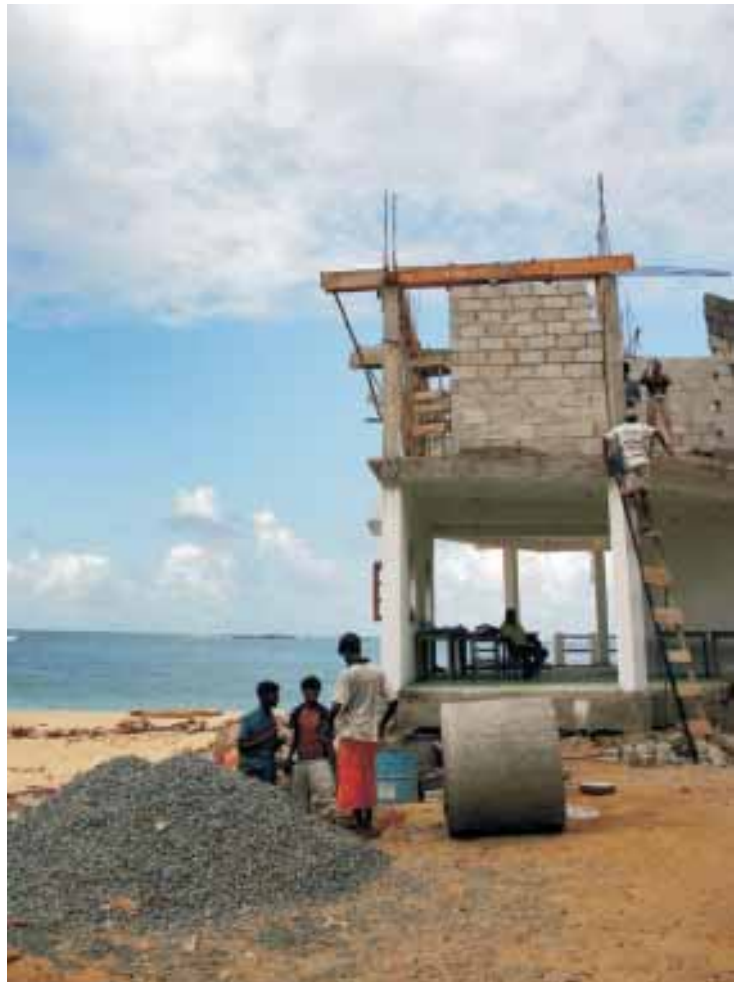
Workers rebuild a small tourist hotel in Unawatuna, southern Sri Lanka. © Anuruddha Lokuhapuarachichi/Reuters
