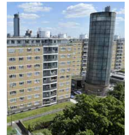
A glass accumulator tower at Pimlico District Heating Undertaking in London stores excess heat from the network.
