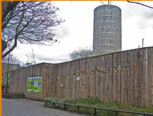
Bunhill CHP plant in Islington, London. The tower is a large heat storage unit that reduces the need to provide heat from the district heating system's backup gas boilers.
