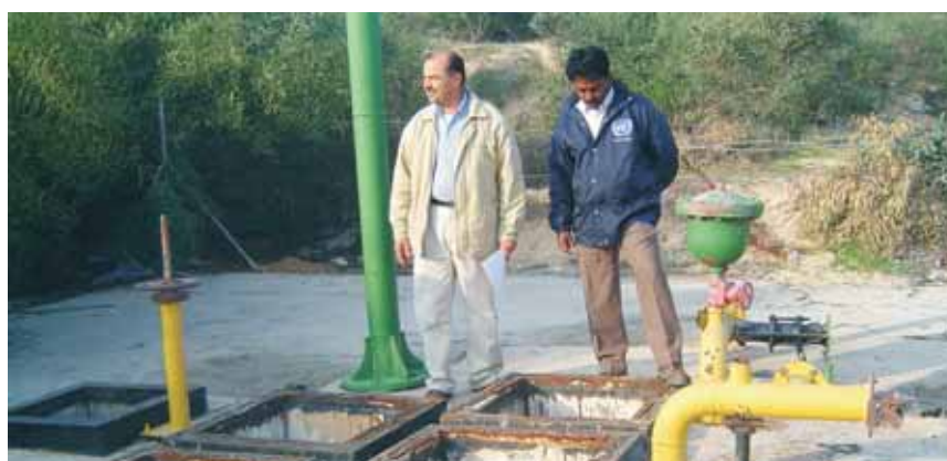
Local and UNEP experts at the site of a subsurface storage tank in Gadid
