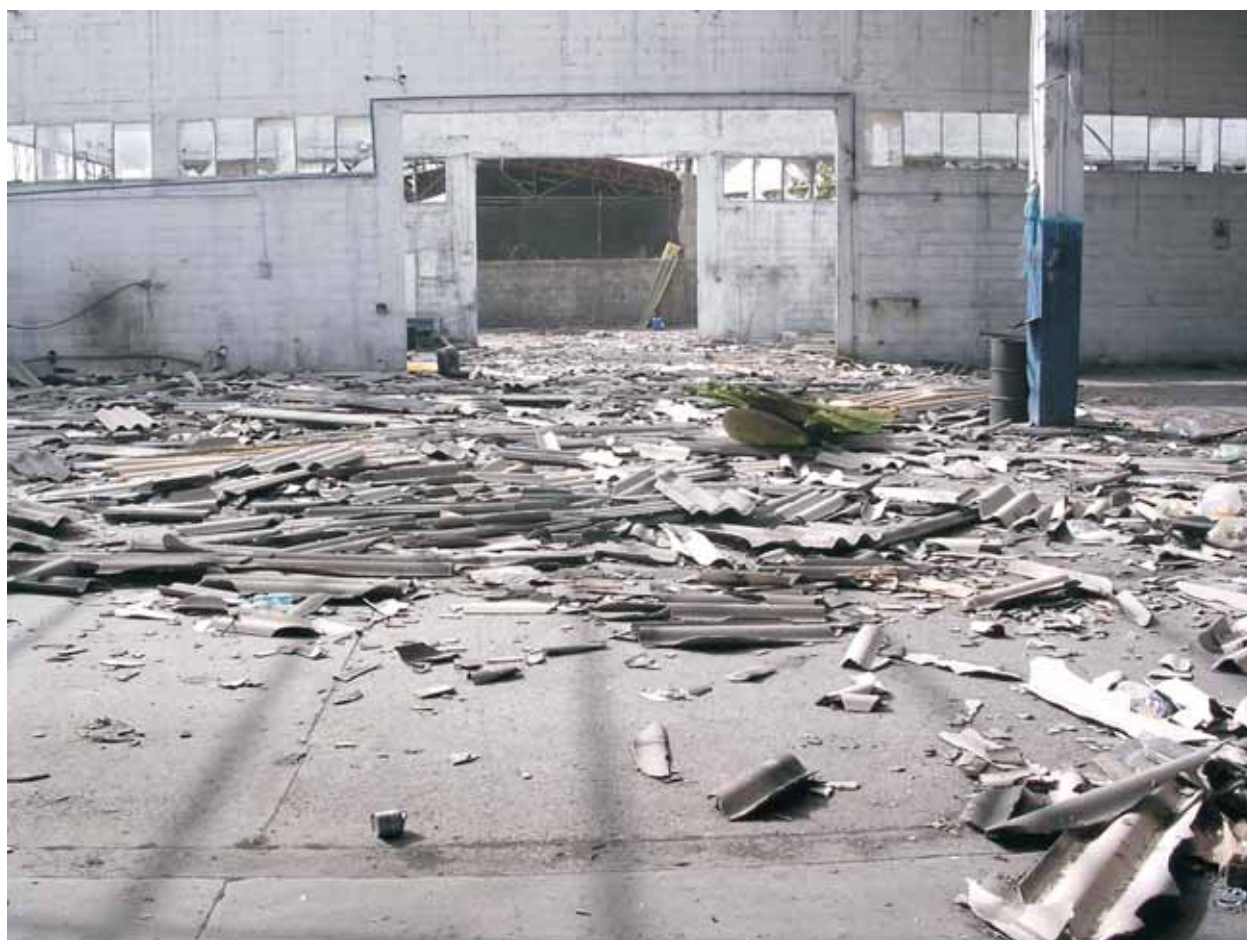
The removal and disposal of rubble remains a major activity to be undertaken prior to resettlement, issues associated with asbestos need to be handled carefully so as not to expose workers to unnecessary harm
