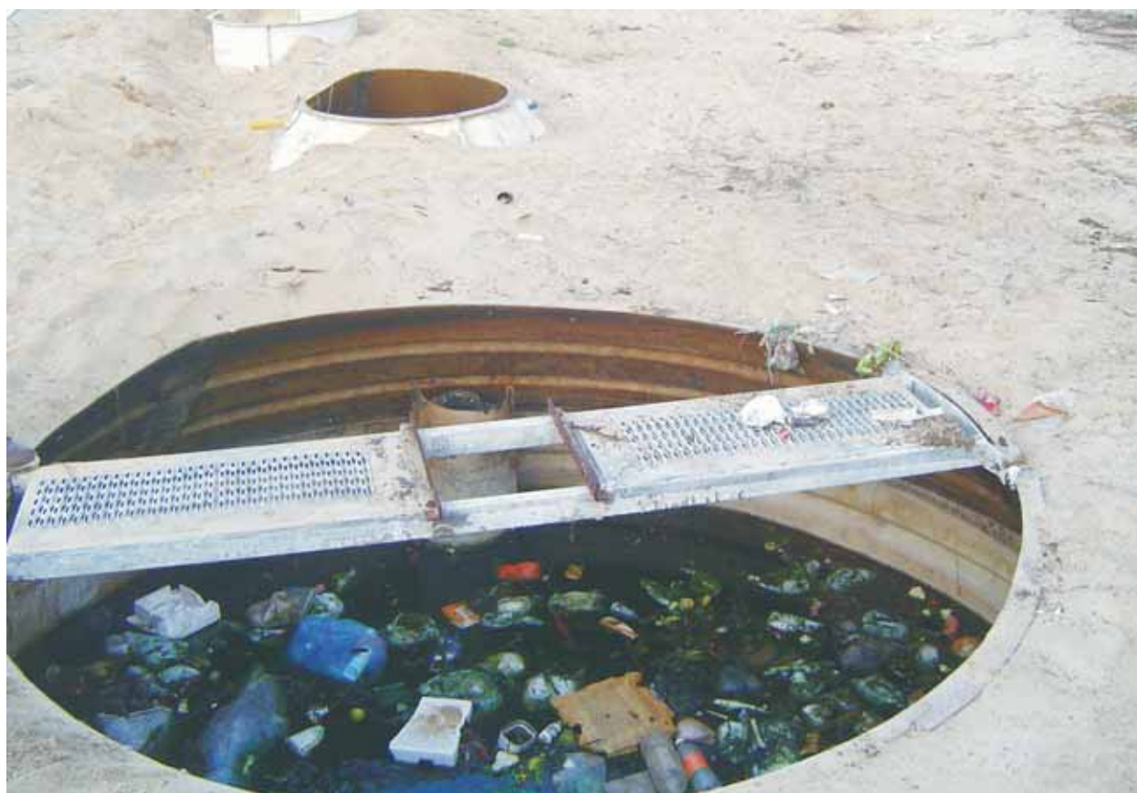
Concrete pit containing accumulated water in the Slav settlement
