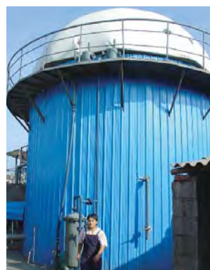
200m 3 integrated biogas plant for animal waste treatment in Badaoshao
