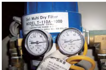
Installation the pressure gauge to measure loss at Multi Dry Filter
