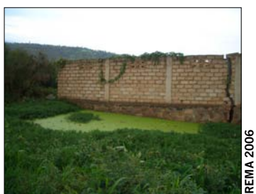
A structure under construction in a wetland is abandoned in the Nyabugogo wetland.
