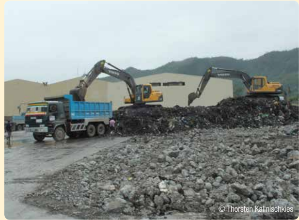
Temporary dumpsite, Tacloban Abucay
