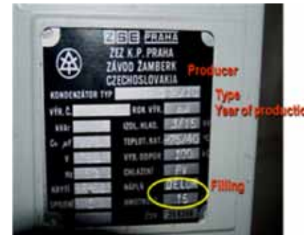
Picture 13: Identification of Capacitor Fluid
