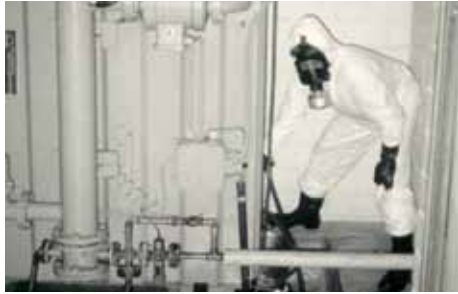
Picture 53: Draining of a PCB transformer
