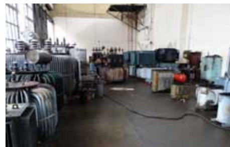
Picture 40: Transformer maintenance area
