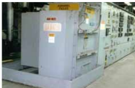
Picture 39: Retention system made from steel
