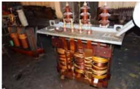
Picture 52: Remains of transformers in a scrap yard
