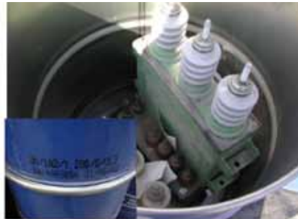
Picture 68: PCB capacitors in steel drum
