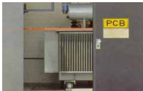
Picture 38: Labelling of a transformer room door
