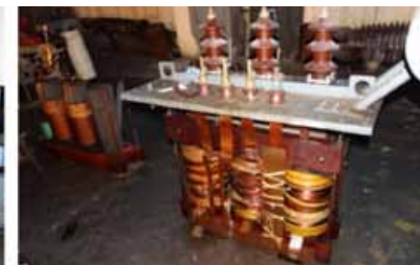
Picture 41: Active transformer part in Albanian workshop
