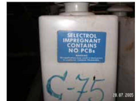
Picture 14: Tag Information on Capacitor
